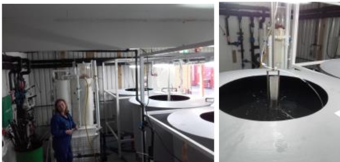
Figure 17.1.1. RAS system and first feeding tanks.
