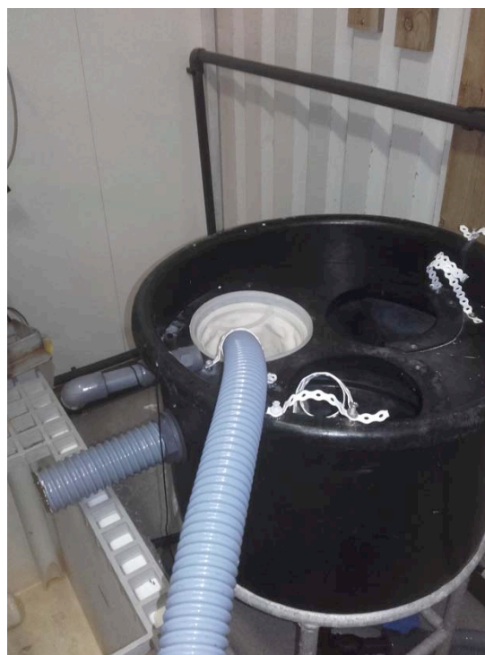
Figure 17.1.6. Bag filter and sedimentation tank.
