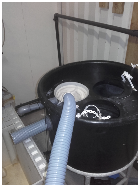
Figure 5. Bag filter and sedimentation tank. Water returned from the larvae tanks and entered the bag filter where large particles and Artemia were removed.
