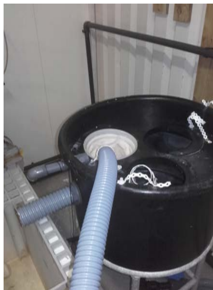
Figure 17.2.7. Bag filter to remove access Artemia and sedimentation tank for clay.
